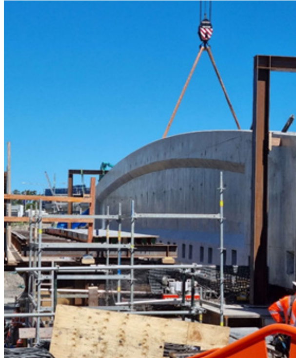
Figure 14 – Photo of the girder restraint system on site.
